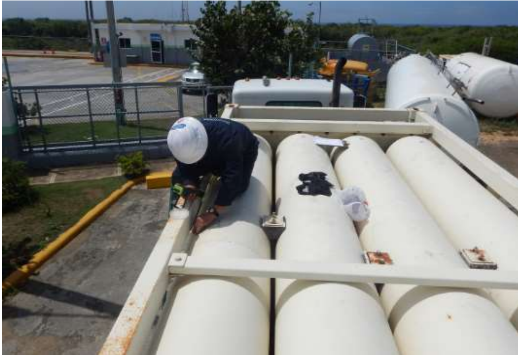
(PDM Group S.A.C Condition Monitoring)
