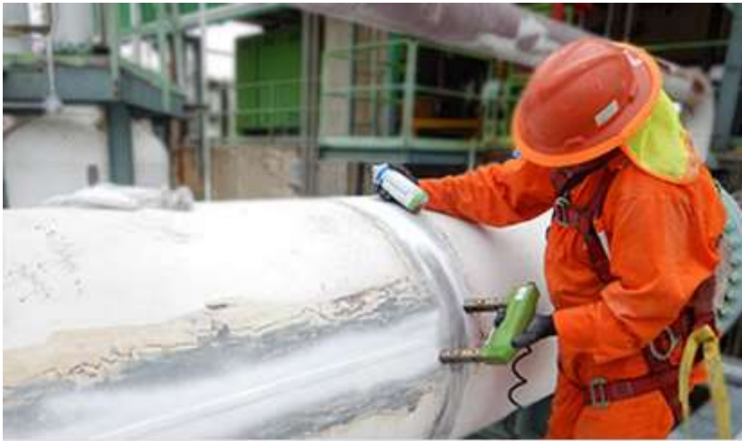
(PDM Group S.A.C Condition Monitoring)
